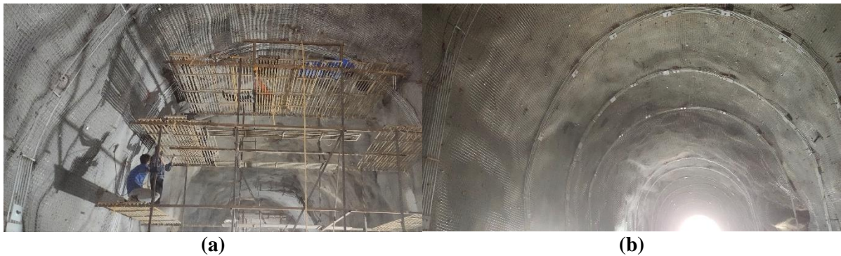
Figure 6. (a) installation of reinforced ribs of sprayed concrete; (b) view of tunnel after installation of RRS.
