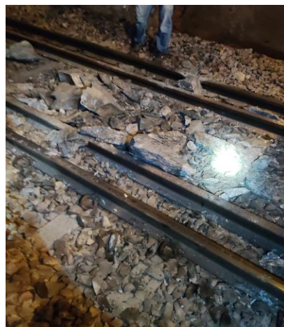
Figure 7. Falling of rock block from the crown of tunnel.
