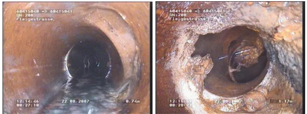
Figure 34. Damage situation in the main sewer (left) and in the area of the house connection spigot with view into the connection sewer (right) [36].
