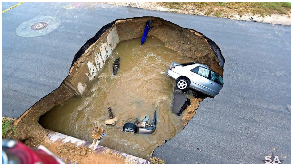
Figure 6. Giant hole in the road [6].
