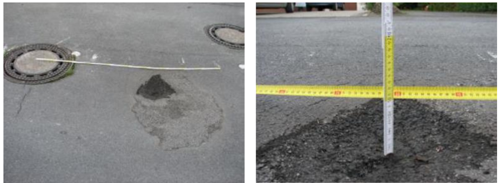
Figure 32. Road damage: Trough-like deformation, breakout, patching [36].
