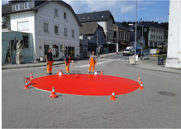
Figure 18. Mini roundabout with a passable central island in the author's place of residence [16,17].
